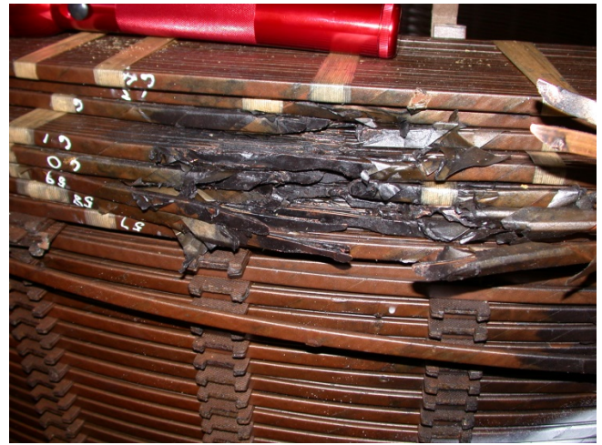
Figure 2: Damage to a large power transformer in South Africa due to the effects of a space weather storm which gave rise to GICs.
