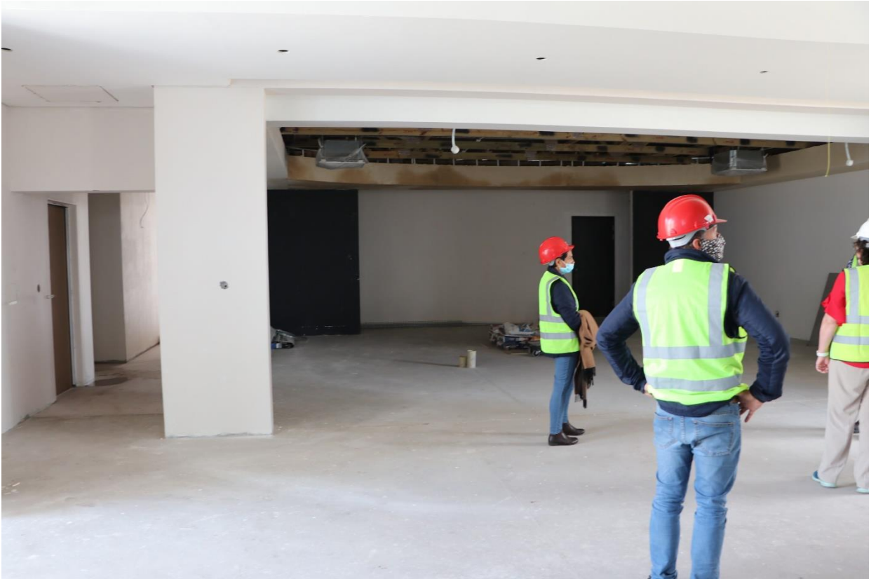
Figure 6 Foyer area looking into Control Room
