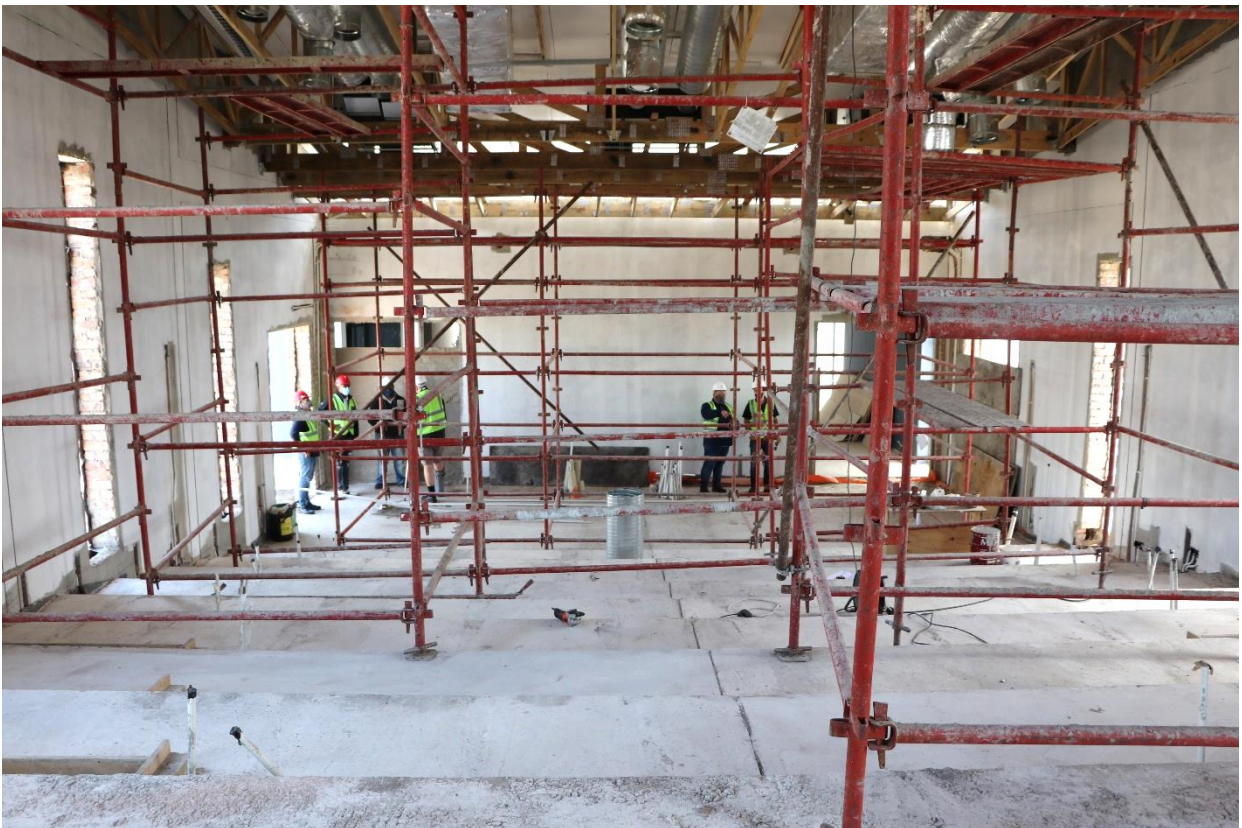
Figure 4 Auditorium view from sound desk to stage
