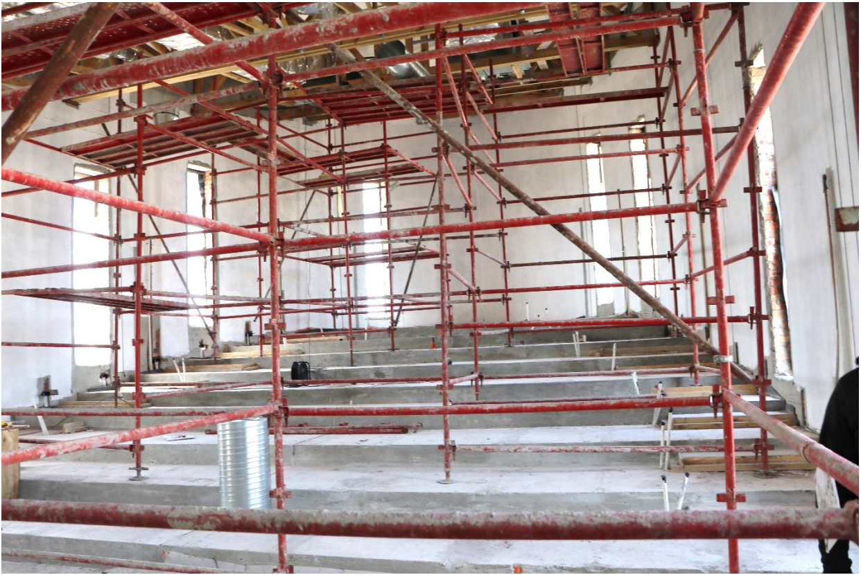
Figure 3 Auditorium view from stage to sound desk
