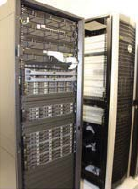
The SANDIMS will essentially control SANSAs instrumentation network used for research and application purposes
